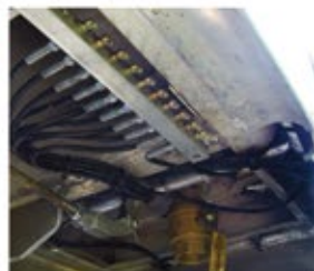
Central Grease Block and Floor Drain Valve
